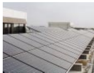
The roof of the offices at the Company's Mie Plant is covered with 360 solar panels with 167W modules.
