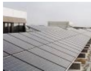
The roof of the offices at the Company's Mie Plant is covered with 360 solar panels with 167W modules.
