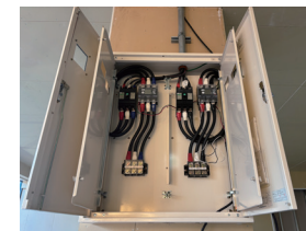
An electricity meter installed in a tenant space of Shonan Mall FILL
