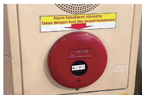
Factory emergency bell
